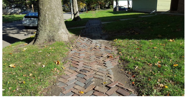
FIGURE 6-11 Brick sidewalk upheaved by tree roots on Elm Street in Historic East Urbana
