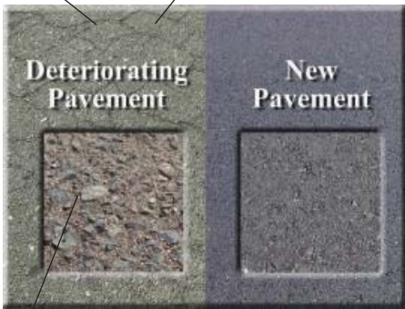
Fine aggregate material loss
