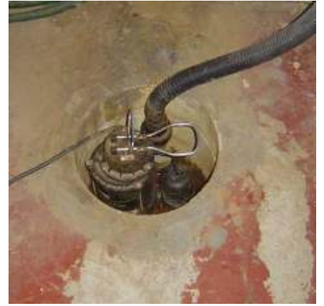
Typical basement sump pump
