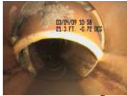
Sewer Televising Showing Collapsed Pipe
