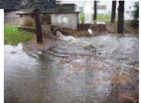
Vine Street Viaduct Pump Station
